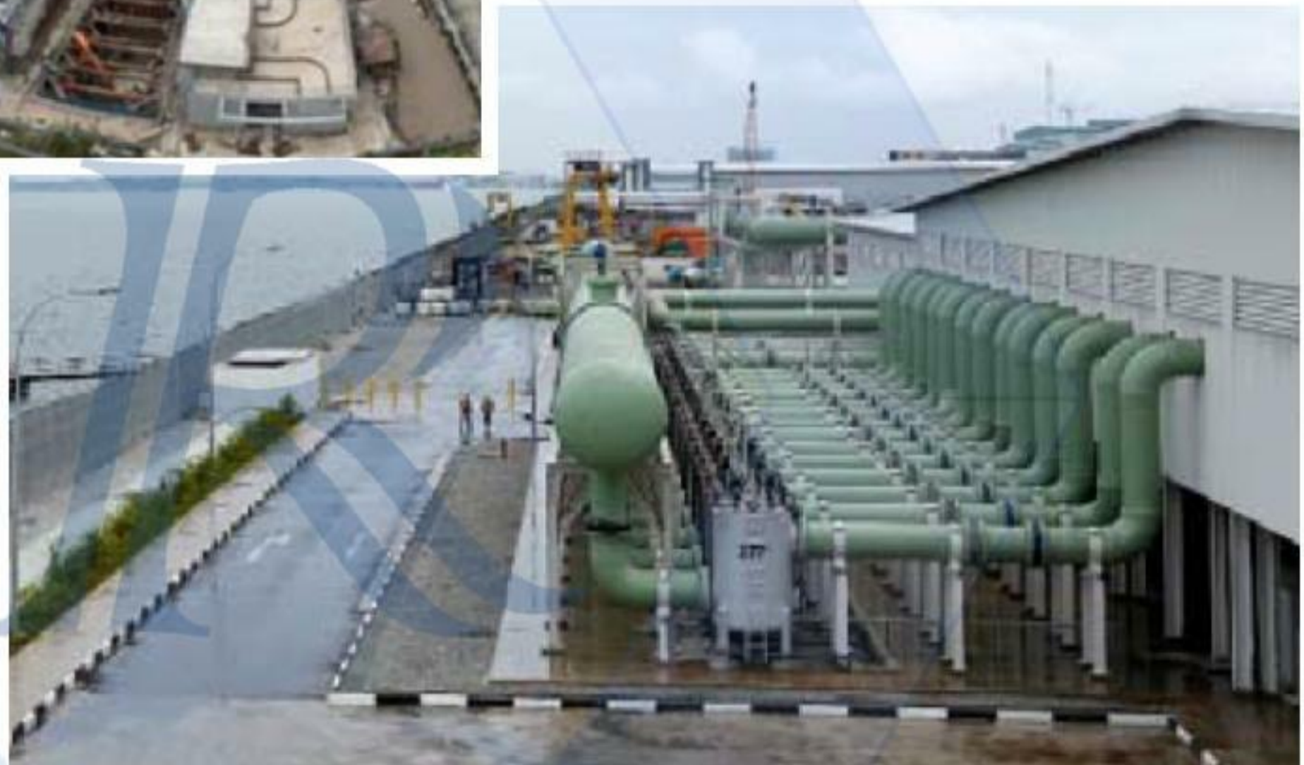
TUAS SPRING DESALINATION PLANT SINGAPORE
